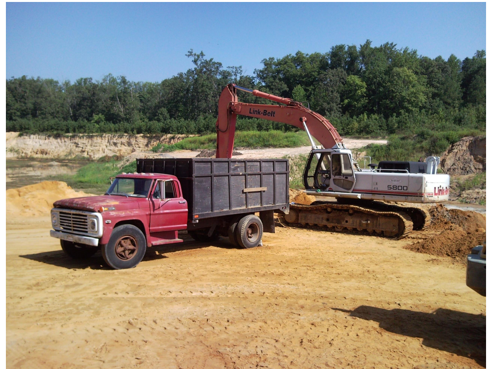
Accident scene after the victim had been removed
